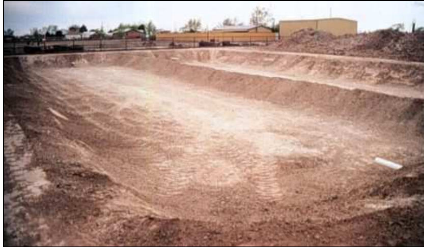
Figure 7. Excavated and graded site showing a slight slope (~1%) in the lengthwise direction of flow (Purdue 2007)
