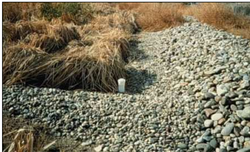
Figure 10. A constructed wetland complete with gravel and vegetation (Purdue 2007)
